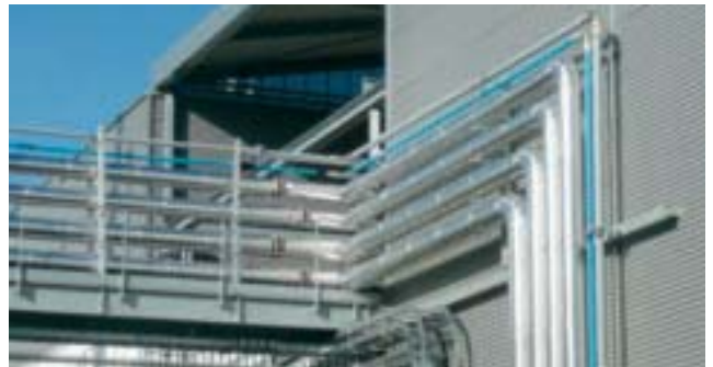
Outdoor installation Transair Ø 168
